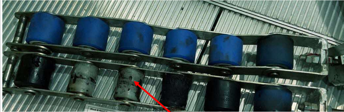
Excessive Wear and Tear
