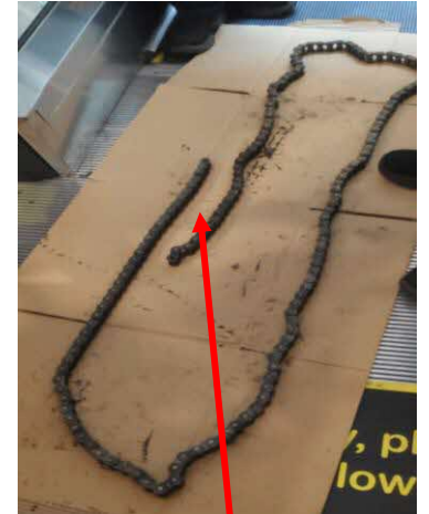
Broken Handrail Drive Chain
